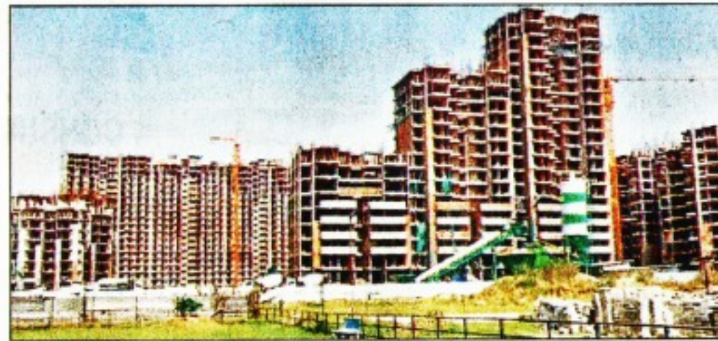
Centurian Park is one of four projects where flats are to be completed
